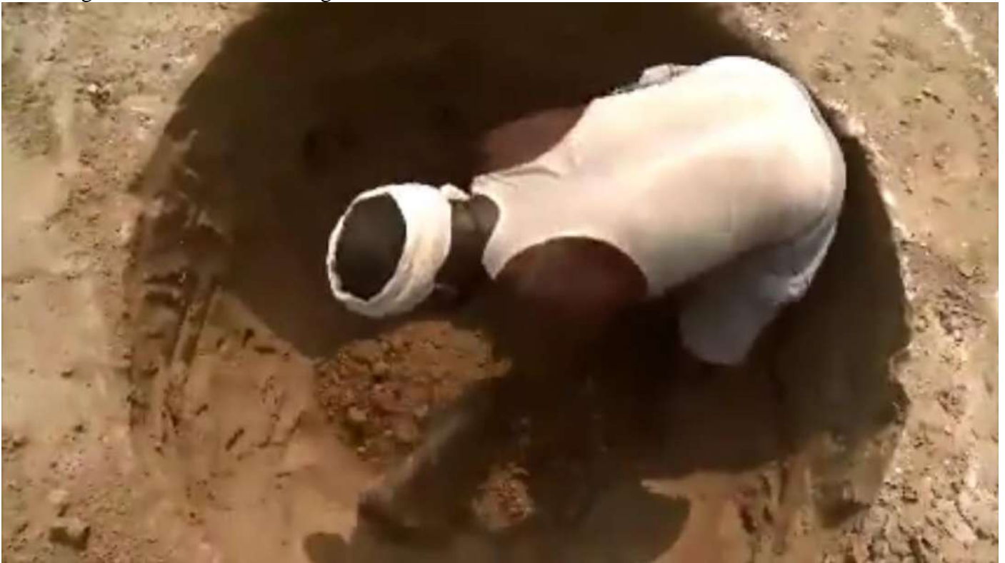
Construction work under progress in a village at Samrala block in Lidhiana.
